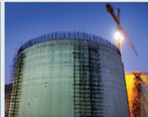
Omidieh Crude Oil Storage
